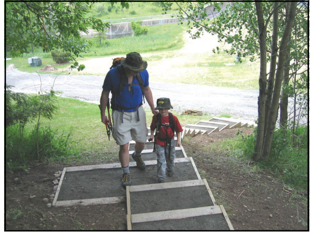
Kirk and Adam Bucynski ascend the newly installed stairway on the Mid State Trail in Hills Creek State Park.
