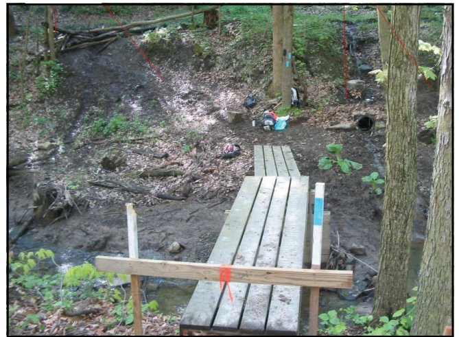
A section of the trail route (to the upper left of the bridge) that has been ground into a muddy, eroded morass by trespassing motorized vehicles. Photo by Dave Brewer.
