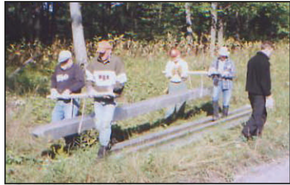
Trail Care Volunteers Move a Bridge Girder to the Work Site. See page 12 for the completed bridge. Photo by Mary Pitzer.
