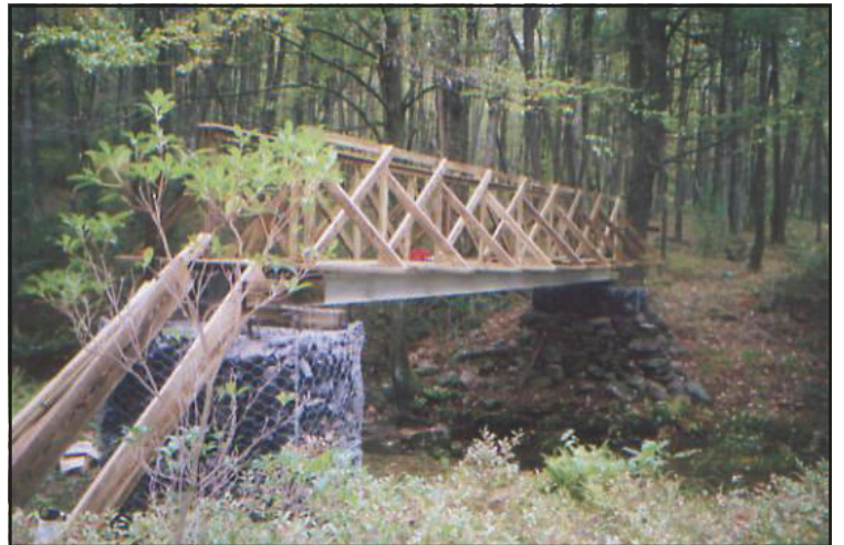
Trail Care bridge on the Chuck Keiper Trail awaits its finishing touches. To see how those girders were transported to the trail site, see page 9. Photo by Mary Pitzer.
