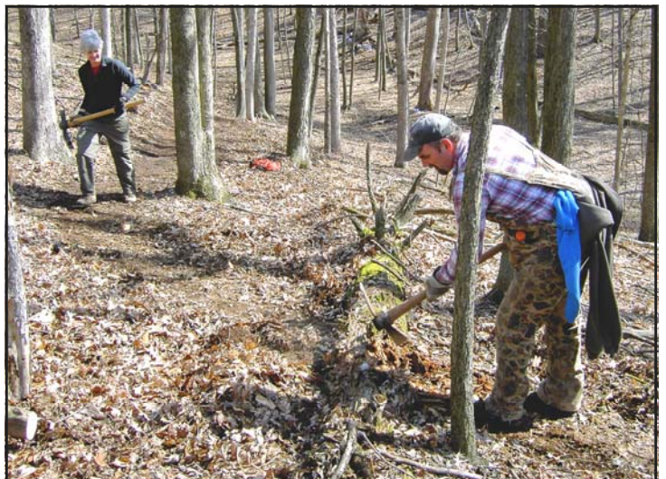
Jen Hollinger and George Gress working on the H-ST reroute at Fort Indiantown Gap on Feb. 21. Photo by John Stein.
